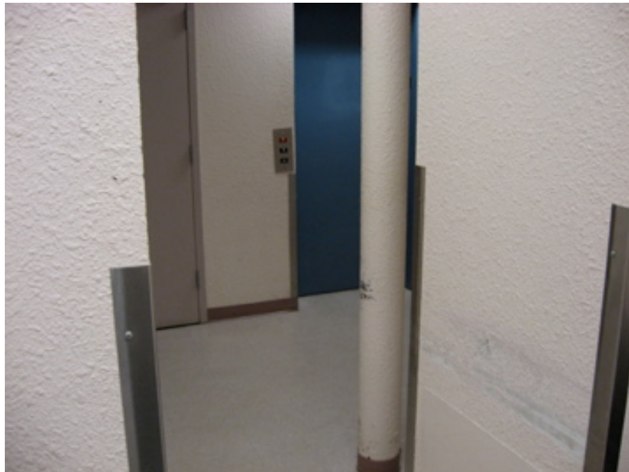
Exhibit F – Hallway Elevator Entrance Blind Spot (Camera Located Around Corner to the Right)
